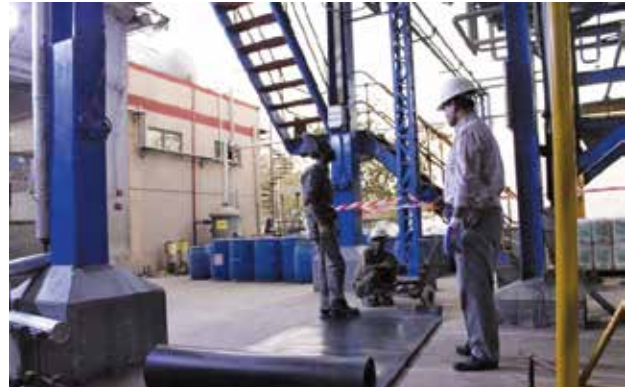
The Chemicals team executes its annual plant shutdown
