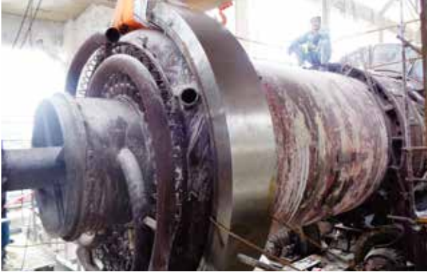
The Soda Ash team successfully replaced the calciner ring at the Soda Ash plant, improving efficiency.
