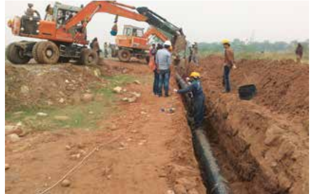
The Soda Ash project team laid a new water pipeline using steel mesh reinforced polyethylene pipe.
