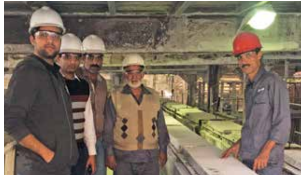
A group of young engineers innovatively replaced the ash conveyor using only in-house resources, upgrading the capacity of the conveyor to 200 tons per day.
